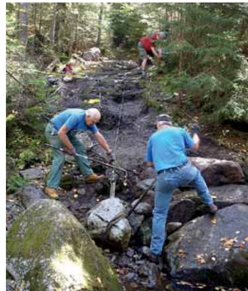
BELOW: VOLUNTEERS FROM THE TRAILWRIGHTS USE A WINCH, CABLE, AND BARS TO GUIDE A ROCK STEP INTO PLACE ON THE MT. KINSMAN TRAIL. A CREW OF FOUR SPENT A TOTAL OF 40 HOURS ON THIS DAY INSTALLING FIVE ROCK STEPS NEAR A STREAM CROSSING. BRUCE RICHARDS PHOTOGRAPH.
