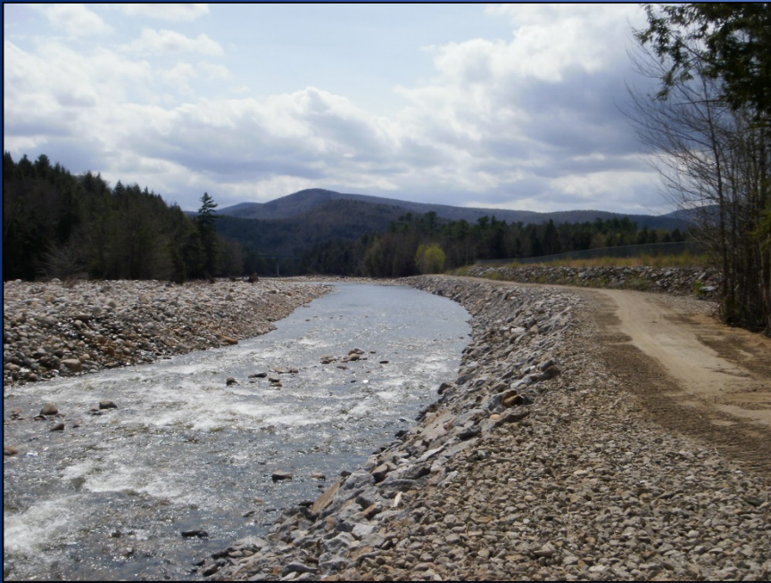
Riprap bank stabilization on the East Branch of the Pemigewasset River adjacent to municipal sewage lagoons in Lincoln, NH
