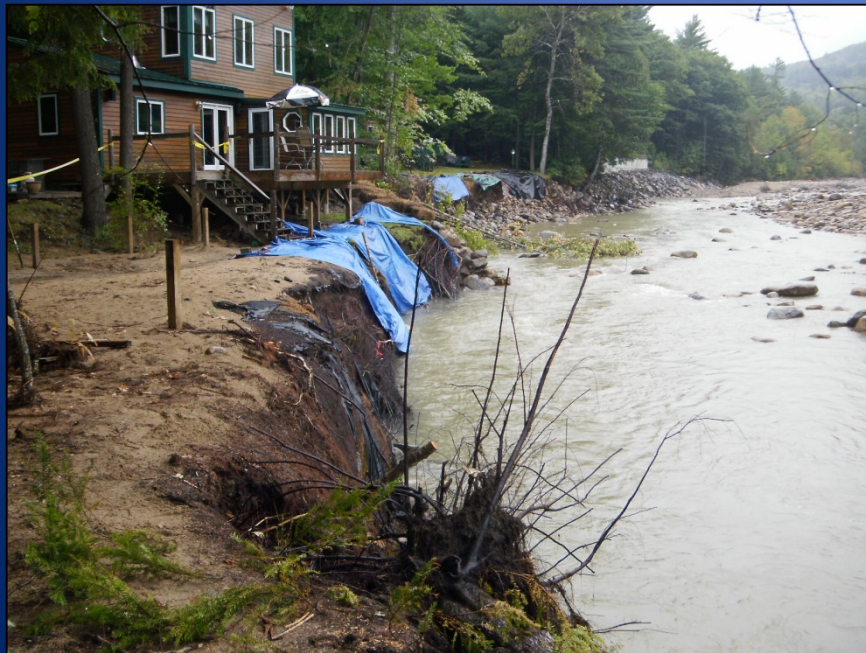
Bank erosion on the Mad River in Campton, NH following TS Irene
