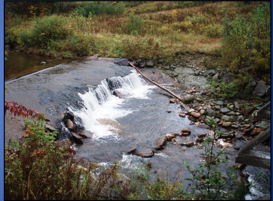
Concrete-encased oil pipeline across Stag Hollow Brook in Jefferson, NH creating a fish passage barrier
