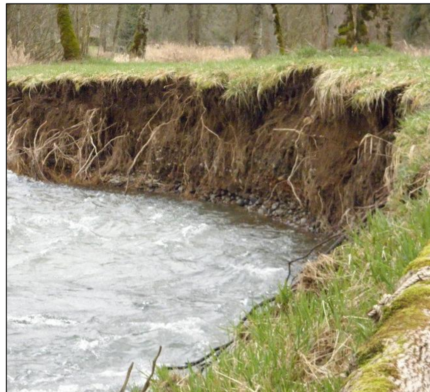
Bank Erosion ( Image Credit )
